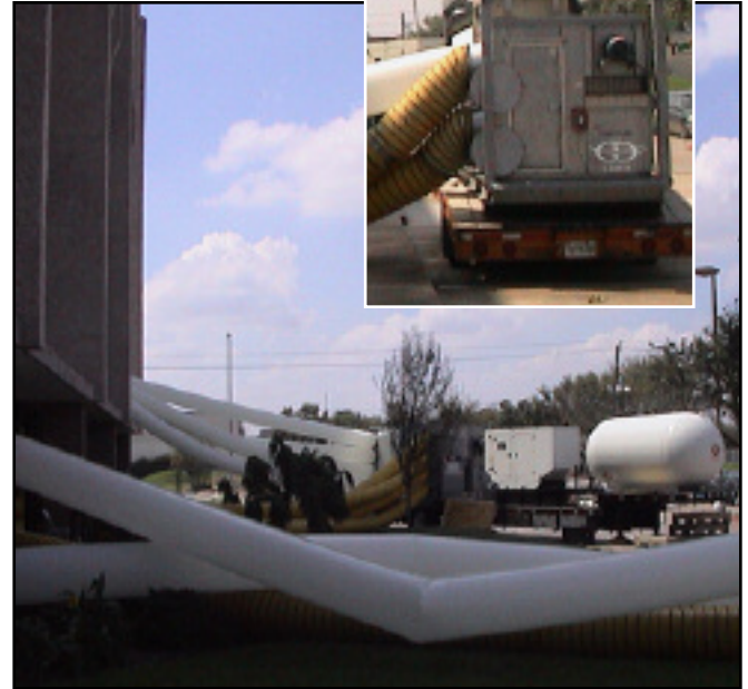
A mobile 25,000 CFM desiccant dehumidifier with generator and a 3,500 gallon propane tank.
